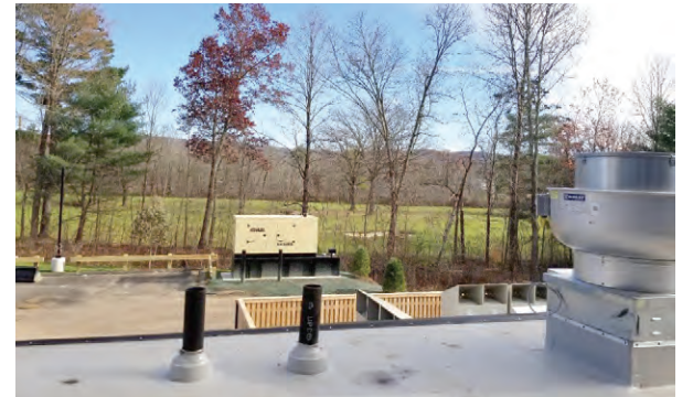
On the second floor, the view to the east shows a County Club fairway. In the near distance is the emergency generator for the Senior Center that has yet to be placed in its permanent home.
