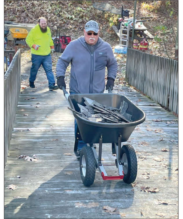
Don Talbot, VFW Post 9397 clerk, hauls old pieces of the pavilion roof as Quartermaster Jered Sasen follows.
