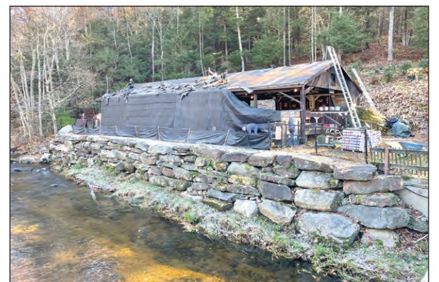
On Nov. 1, a team of volunteers gathered to repair the roof at VFW Post 9397.
