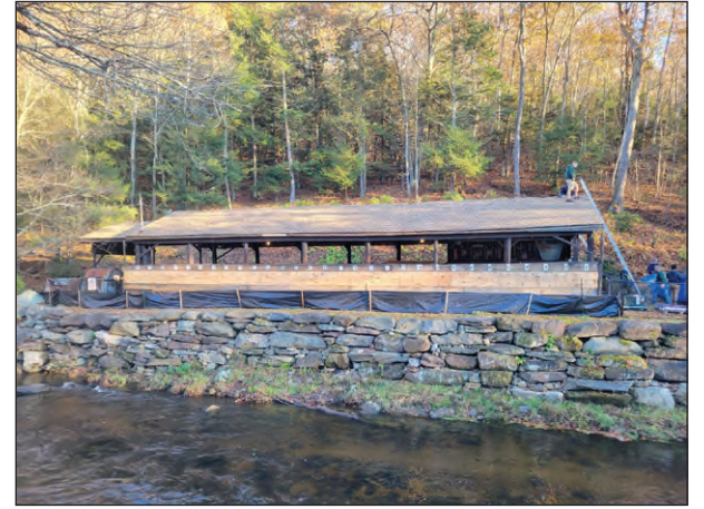
Following a significant volunteer effort, the VFW Post 9397 pavilion has a new roof. Photo courtesy of Jered Sasen, VFW.
