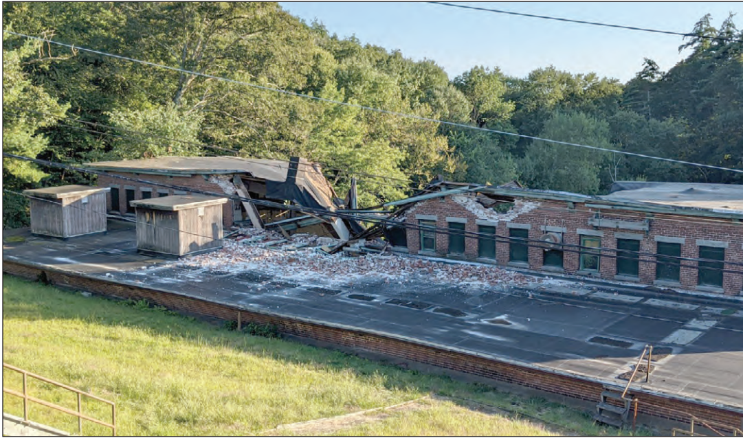
A close-up of the damage after the collapse and fire at the Red Bridge Hydro Plant on Red Bridge Road on Aug. 22. The investigation into the cause of the collapse and fire is ongoing.
