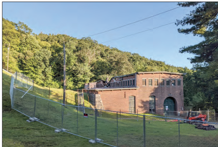
A full shot of the Red Bridge Hydro Plant on 5 Red Bridge Rd. which experienced a building collapse and small fire on Aug. 22.
