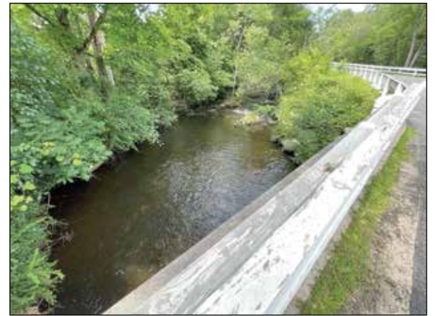
The bridge on Rock-A-Dundee Road will receive state funding for repairs.
