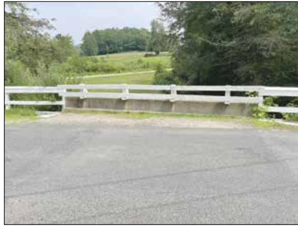
The state will replace the makeshift fence on the sides of the Rock-A-Dundee Road bridge.
