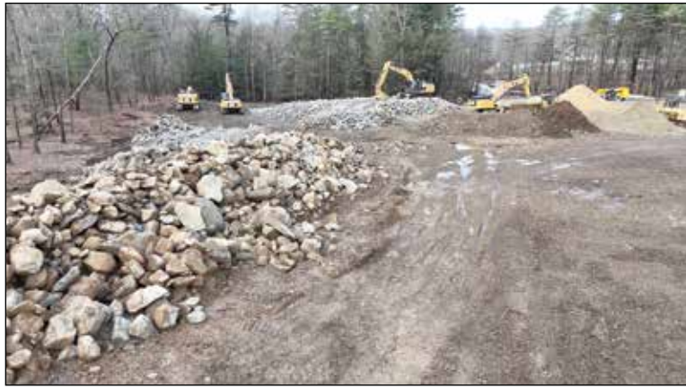
A shot of construction vehicles working with piles of boulders and dirt in the construction area of the 285 Three Rivers Rd. solar project.
