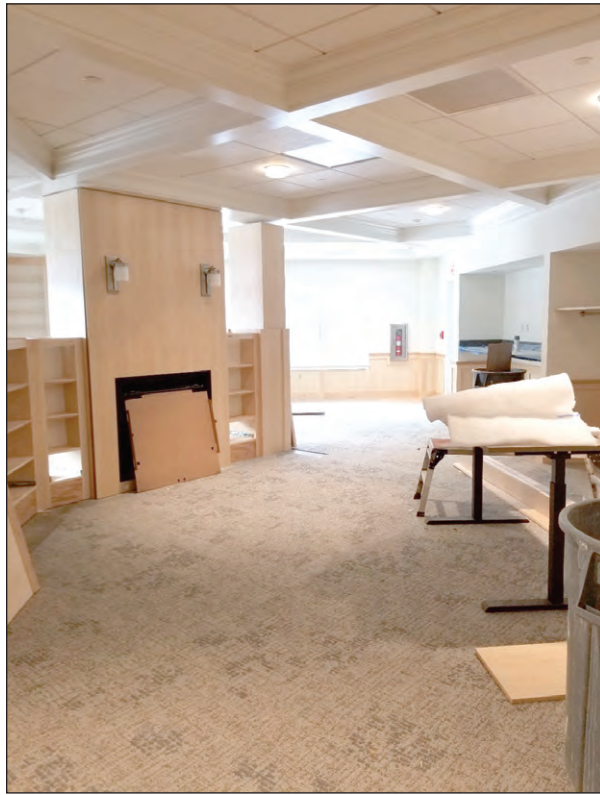
And for those chilly days when you just want to curl up with a good book, the library is taking shape!! Check out the ceiling details!
